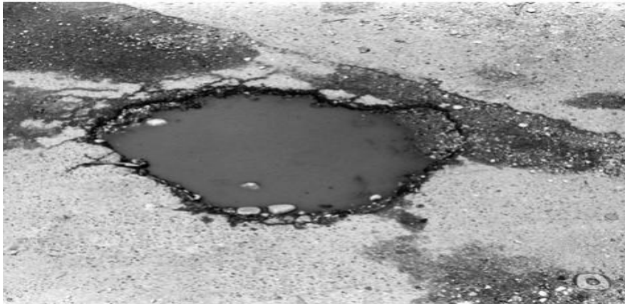
Figure 2. Potholes deterioration (Ahmad & Khawaja, 2018).
