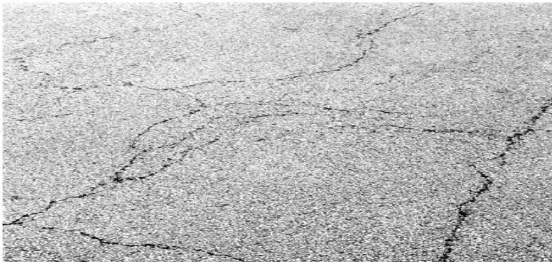
Figure 4. Block cracks Deterioration (Bukhari & Aman, 2023)
