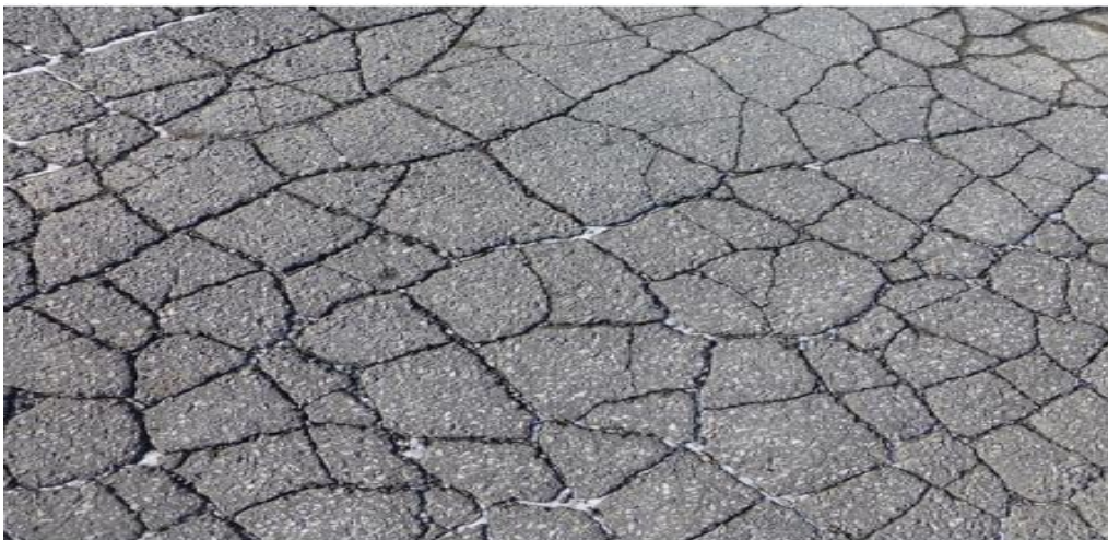
Figure 5. Shows Fatigue cracks and Deterioration (Ahmad & Khawaja, 2018)
