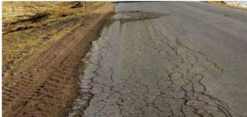
Figure 3. Edge cracks: Deterioration (Chai et al., 2023)
