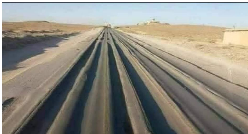
Figure 1. Deterioration of the Kabul-Kandahar highway (Google, 2019)
